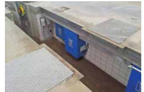
hydraulic pump unit in pit (VLTWPD9752)
